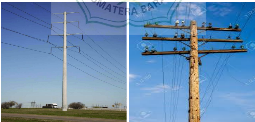
(c) Concrete Pole
