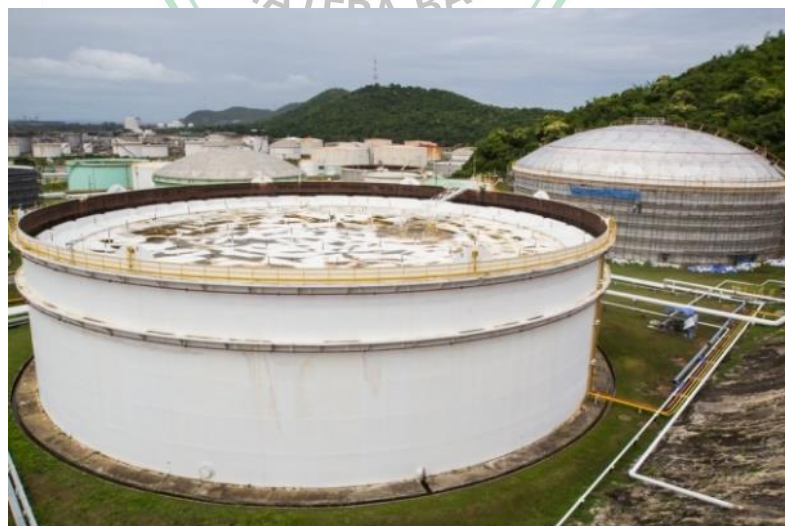
Gambar 2. 5 Floating roof tank.
