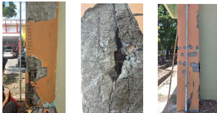
Pic 1 – Condition of the 1st-floor column of the Rectorate Building, Muhammadiyah University of Sumatera Barat (Personal documentation, 2024)
