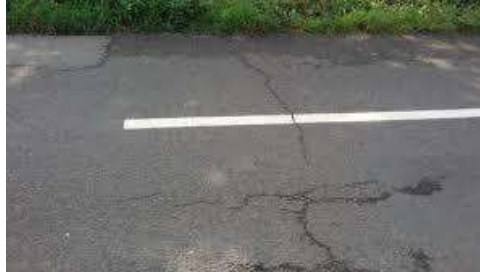
Gambar 2.11 Retak Melintang ( Transversal Cracks )
