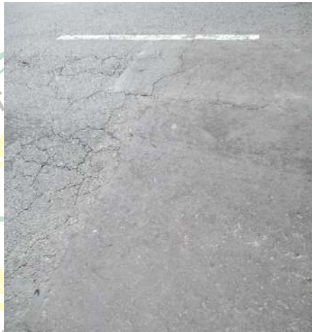
Gambar 2.3 Retak Halus ( Hair Cracking )
