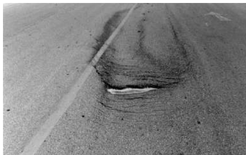
Gambar 2.10 Retak Selip ( Slippage cracks )
