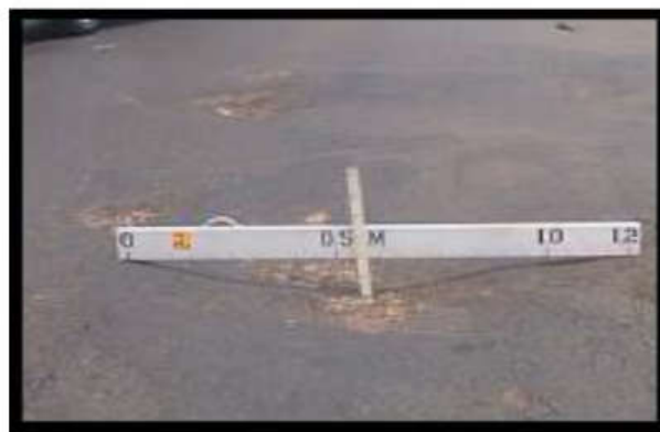
Gambar 2.9 Amblas ( Depression ) (Sumber : Bina marga no. 03/MN/B/1983 )
