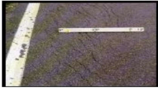
Gambar 2.16 Retak Slip ( Slippage Cracking )
