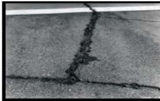
Gambar 2.11 Retak Sambung ( Joint Reflection Cracking )
