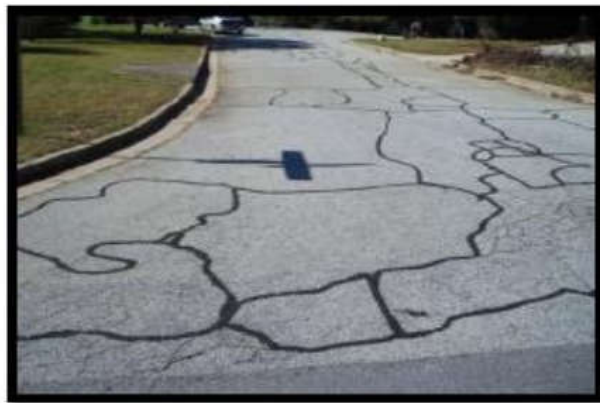
Gambar 2.5 Retak Balok ( Block Cracking ) (Sumber : Bina marga no. 03/MN/B/1983 )
