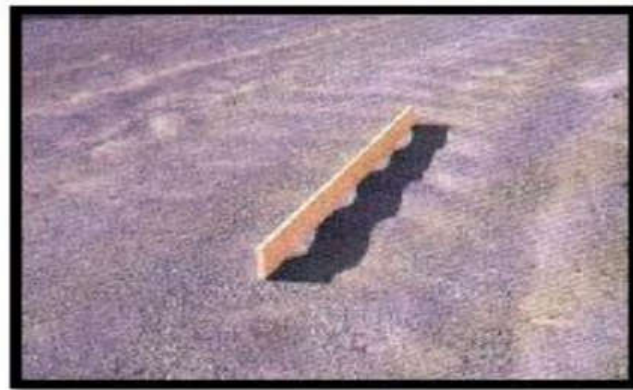
Gambar 2.8 Retak Keriting ( Corrugation Cracking )
