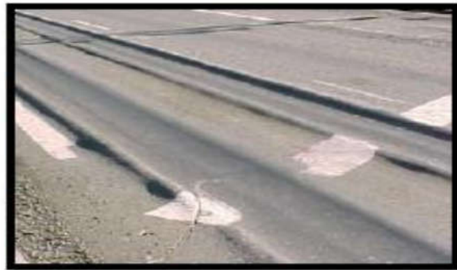
Gambar 2.17 Retak Alur ( Rutting ) (Sumber : Bina marga no. 03/MN/B/1983 )
