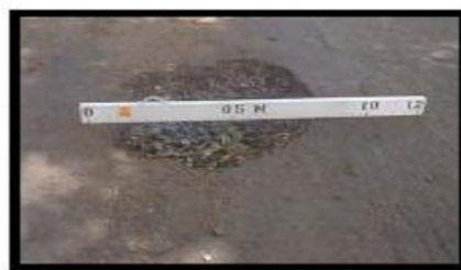
Gambar 2.11 Lubang ( Potholes ) (Sumber : Bina marga no. 03/MN/B/1983 )
