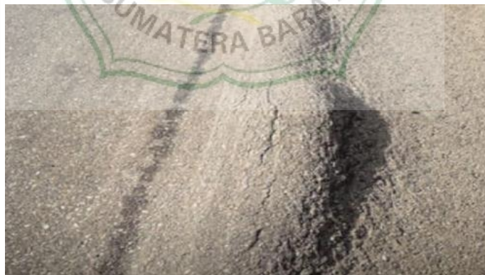
Gambar 2.9 Retak Sungkur ( Rutting ) (Sumber : Bina marga no. 03/MN/B/1983 )
