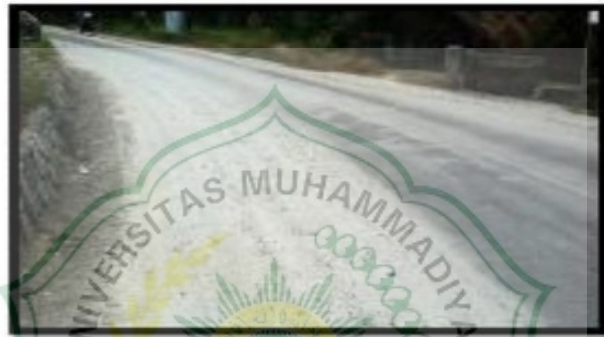
Gambar 2.10 Pelepasan Butir ( Weathering/Raveling ) (Sumber : Bina marga no. 03/MN/B/1983 )
