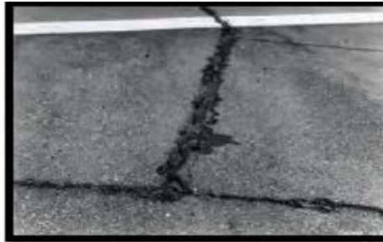
Gambar 2.7 Retak Sambung ( Joint Reflection Cracking ) (Sumber : Bina marga no. 03/MN/B/1983 )
