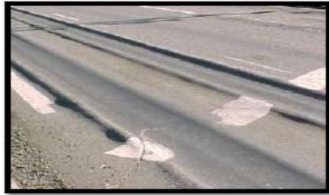
Gambar 2.8 Retak Alur ( Rutting ) (Sumber : Bina marga no. 03/MN/B/1983 )
