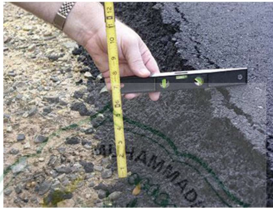
Gambar 2.17 Kerusakan Jalan Lane / Shoulder Drop Off
