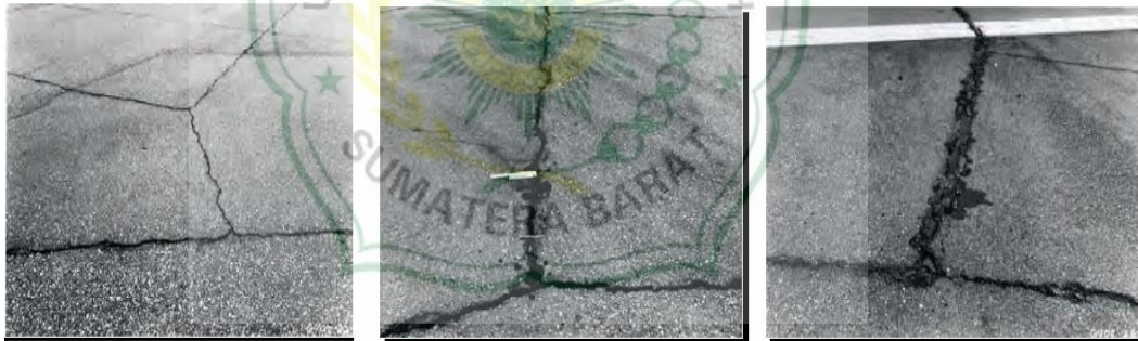
Gambar 2.4 Kerusakan Jalan Joint Reflection cracking Low Severity, Medium Severity dan High Severity
