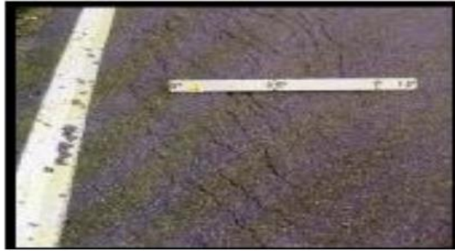
Gambar 2.16 Retak Slip ( Slippage Cracking ) (Sumber : Bina marga no. 03/MN/B/1983)
