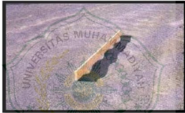
Gambar 2.8 Retak Keriting ( Corrugation Cracking ) (Sumber : Bina marga no. 03/MN/B/1983)
