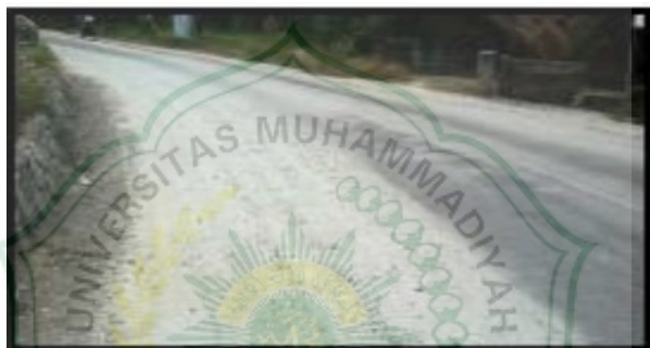
Gambar 2.18 Pelepasan Butir ( Weathering/Raveling ) (Sumber : Bina marga no. 03/MN/B/1983)
