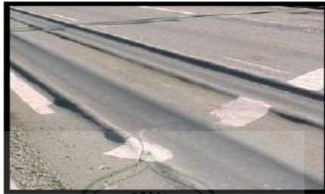
Gambar 2.17 Retak Alur ( Rutting ) (Sumber : Bina marga no. 03/MN/B/1983)
