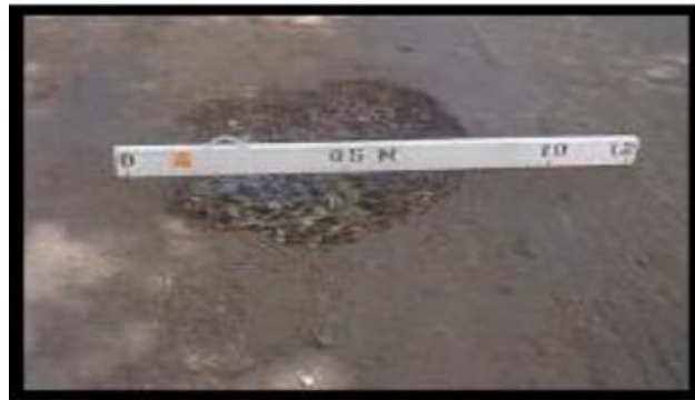
Gambar 2.15 Lubang ( Potholes ) (Sumber : Bina marga no. 03/MN/B/1983)
