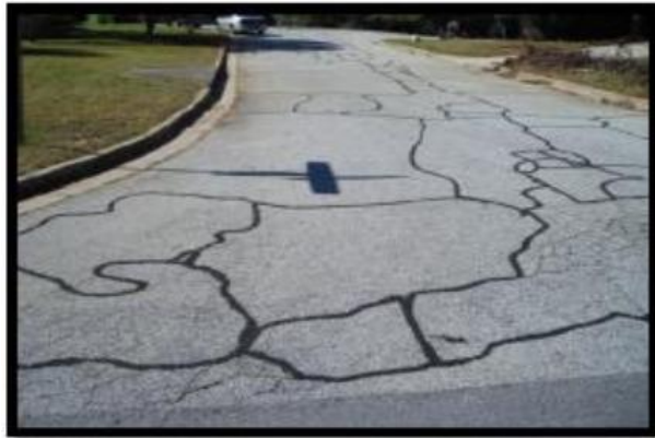
Gambar 2.4. Retak Blok ( Block Cracking ) (Sumber : Bina marga no. 03/MN/B/1983)
