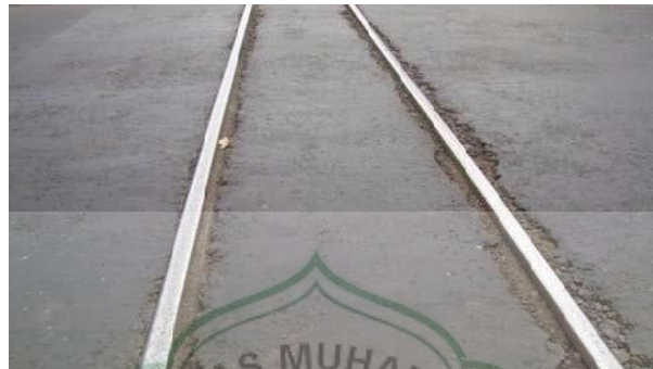
Gambar 2.14 Rusak Perpotongan Rel ( Railroad Crossing )
