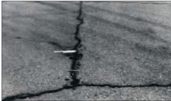
Gambar 2.8 Retak Sambung ( Joint Reflection Cracking )
