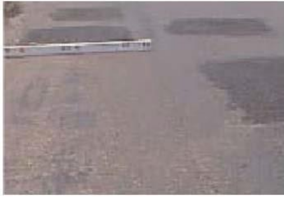
Gambar 2.11 Tambalan ( Patching and Utility Cut Patching ) Sumber : Google (2021)
